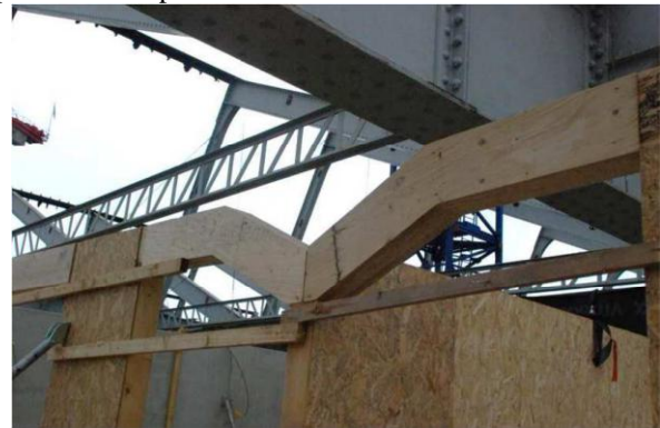
Figure 13: The new wood structure is totally independent from the existing steel structure / Source : Arbonis
