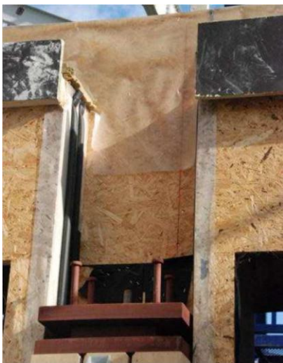
Figure 18: Typical case of the column within the nonbearing façade timber wall / Source Arbonis
